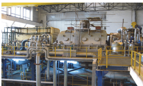
Figure 2. Electricity generator and steam turbine, 150 MW group
