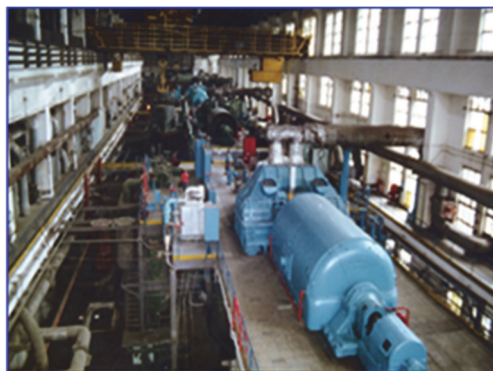
Figure 1. Electricity generator and steam turbine, 50 MW group
